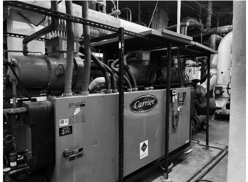
Figure 1, Jones Tower chiller to be removed as part of the project
